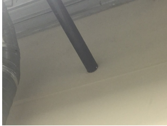
Figure 4: The fire sprinkler main runs perpendicular to adjoining bays. There is no gap; the wall is flush up to the pipe. Photo courtesy of Gladstein, Neandross & Associates, NREL
