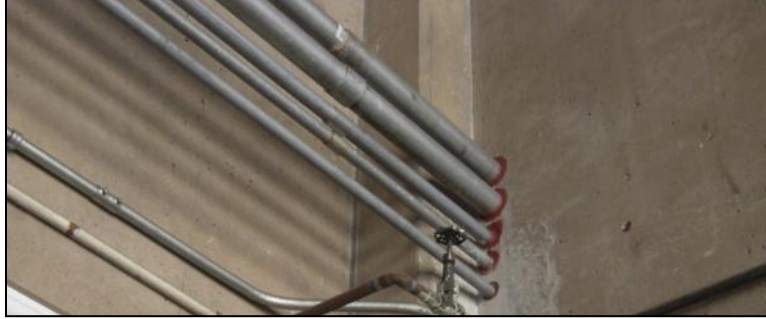
Figure 6: Wall penetrations properly sealed to prevent migration. Photo courtesy of Gladstein, Neandross & Associates, NREL
