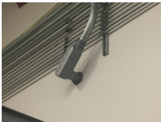
Figure 3: Electrical conduit going into the wall of an all hydrogen service bay is sealed to prevent hydrogen from entering. Photo courtesy of Gladstein, Neandross & Associates, NREL
