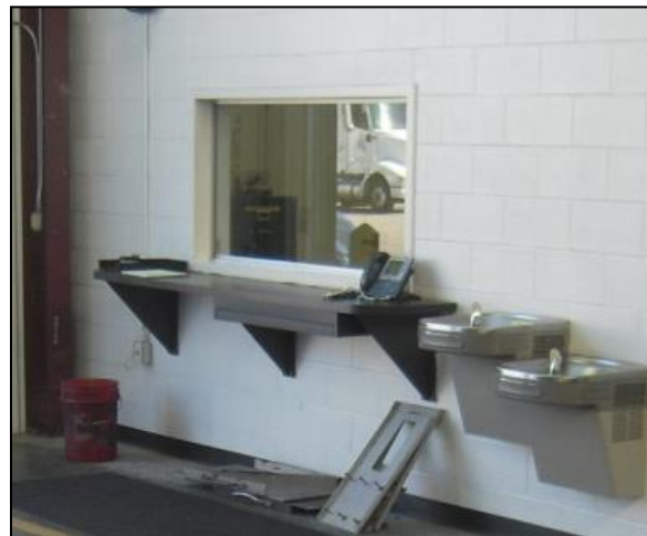
Figure 9: A pass-through window presents a potential path of migration. Photo courtesy of Gladstein, Neandross & Associates, NREL
