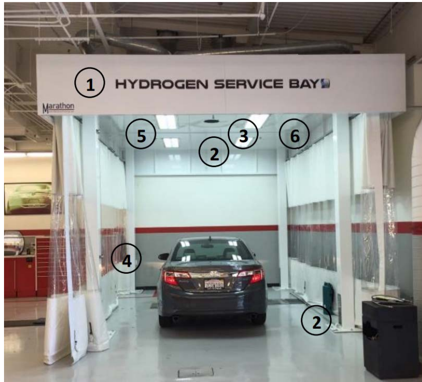
Figure 12: Hydrogen Service Bay, Annotation descriptions below. MarathonSprayBooths.com
